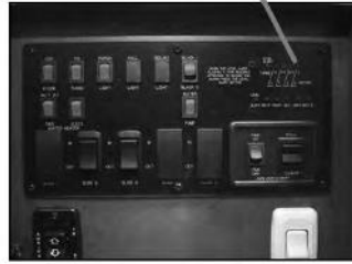
Monitor panel and command center panel
