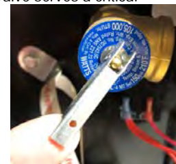
Water Heater Pressure Valve
