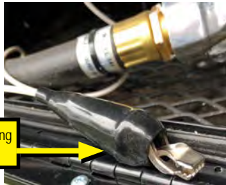
Grounding Clip Inside Fuel Station
