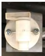
Exterior Fresh Water Drain Example
