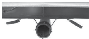
Black/Grey Tank Drain and Valves
